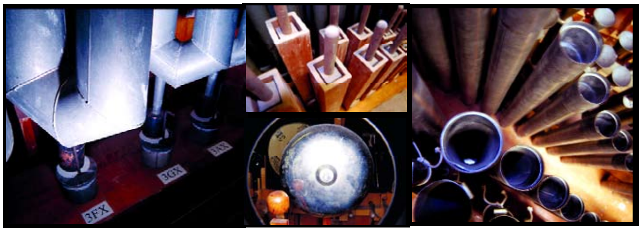
The O'Brien Theatre organ in Renfrew sits behind the movie screen and takes up three floors of the building and part of the basement
